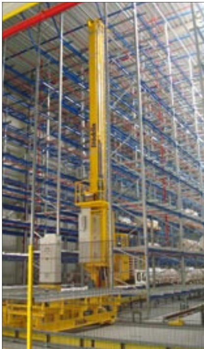
A new fully automatic stock system for raw material storage in the just-completed second production hall
